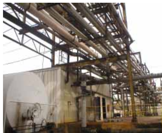
Steam tracing will keep pipes like these from freezing during cold months.
