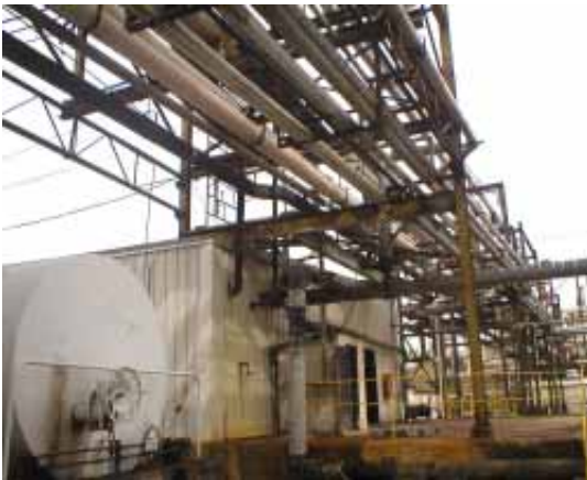
Steam tracing will keep pipes like these from freezing during cold months.
